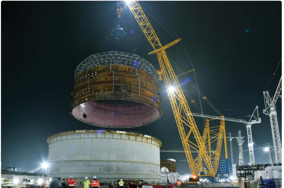
'Big Carl', the world's biggest crane, does the heavy lifting during construction of Hinkley Point C
