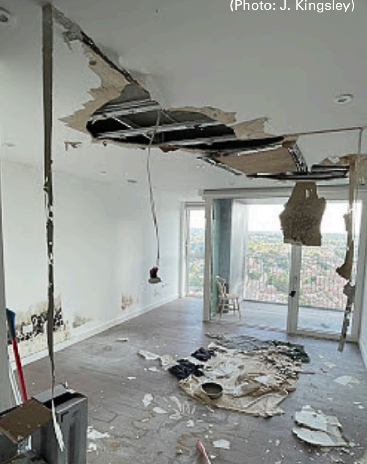
These new flats have water leaks, structural issues and exorbitant rental fees.
